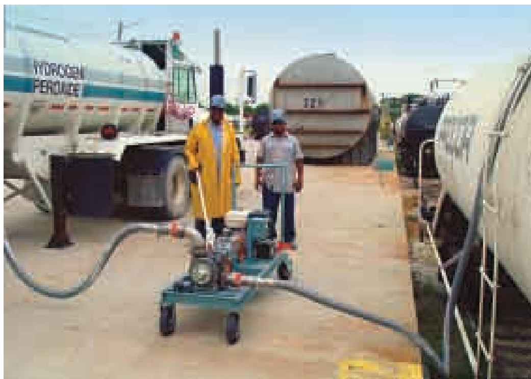
Operators at this chemical distribution/storage terminal facility transloading hydrogen peroxide from a railcar
